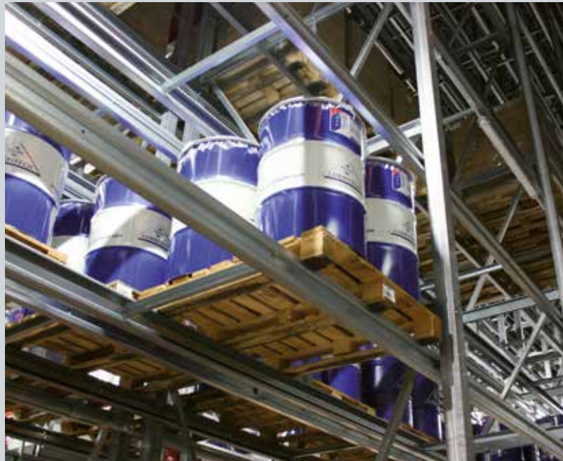
Products with different hazardous material classes under one roof – all safely protected against fire risks
